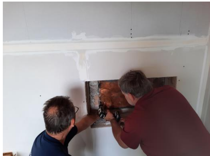
Mike Poole and Brad Dahn sealed the time capsule back up after putting everything back in. The cornerstone will be replaced when the project is complete.
