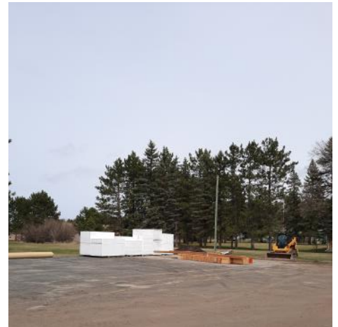
Materials staged and waiting to be installed. Looking forward to walls and windows!
