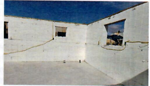
Channels are carved into Styrofoam for electrical wiring. The walls will be stuccoed.
