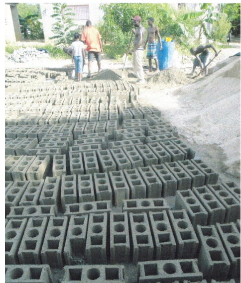
Concrete blocks being made for the construction of the school wall summer/fall 2013. Concrete blocks take several days to make. They are made with a form then watered for several days to harden.
